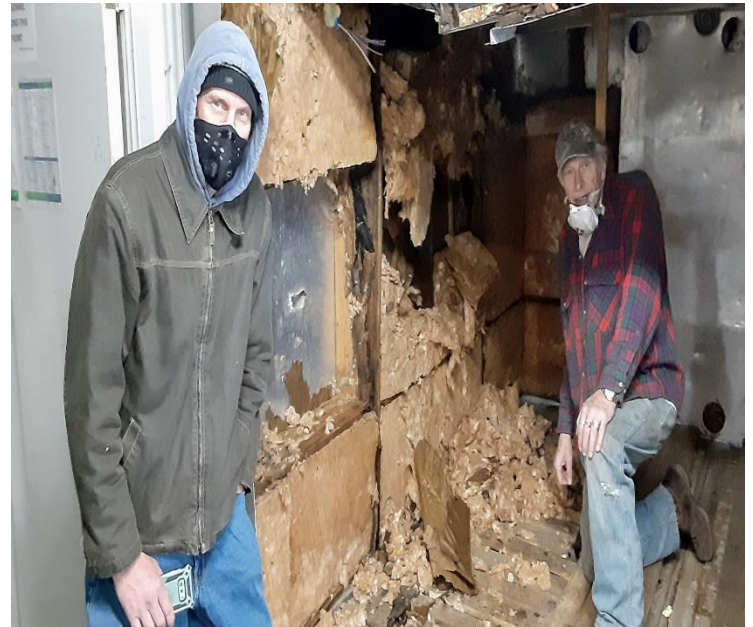
Tearing out all the insulation of the old cooler. A LOT OF HARD WORK had already been done to get to this point of the process.
