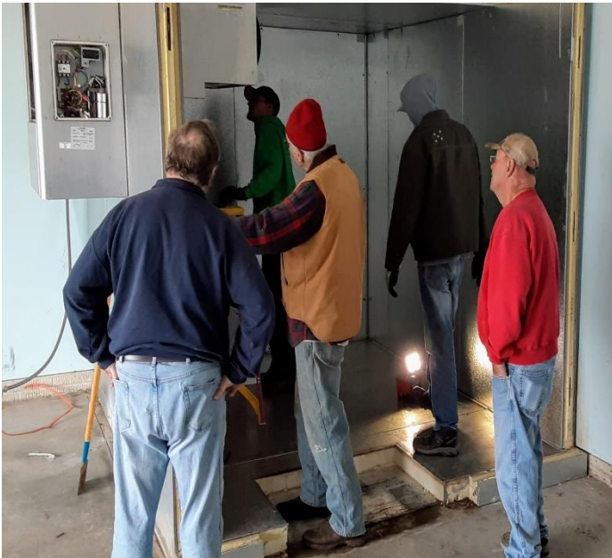
Carefully taking apart the donated walk-in cooler piece by piece and marking each section for assembly at the Fairgrounds.
